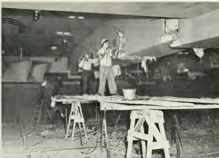
IN REVAMPING NBC'S FAMOUS CONCERT STUDIO 8-H, WORKMEN REMOVE CEILING BEAMS TO MAKE WAY FOR A STEEL OVERHEAD CONSTRUCTION.
