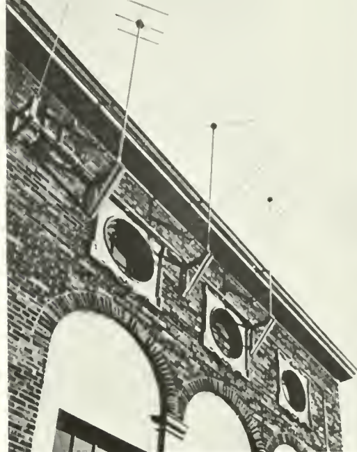
ANTENAPLEX INSTALLATION ON PARK LANE HOTEL IN NEW YORK.
