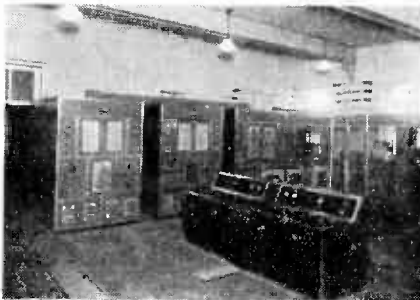
Two of the Italian shortwave transmitters are shown here. To the left is the 43-meter station and next to it is the one which works on 49.3 meters. In the center is the 5 kilowatt panel and at the right are the water-cooled output tubes which raise the power to 20 kilowatts in the aerial.
