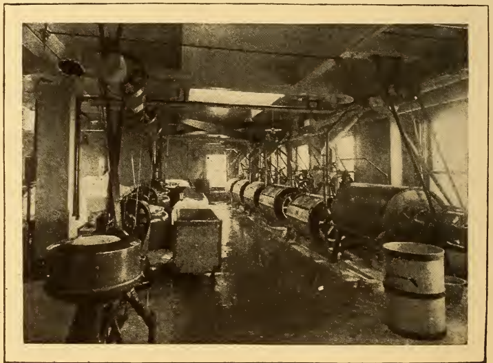
HOW ELECTRICITY IS USED IN THE LAUNDRY OF THE HOTEL ST. FRANCIS
