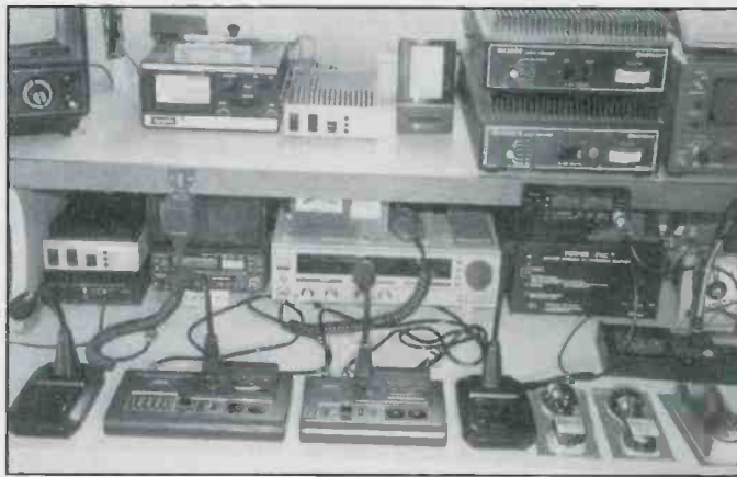
Not all Red Cross radio systems require a ham license to operate. They may also use business band radios.
