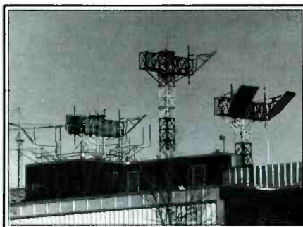
This photo, taken by Patrick M. Griffith, CO shows some of the HF, VHF, and microwave antennas at the Denver Air Traffic Control Center in Longmont, CO.
