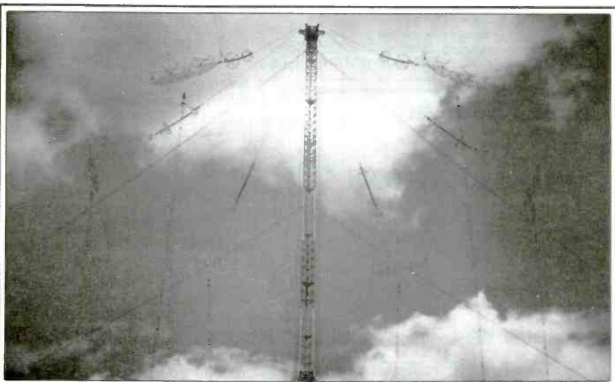
Atop each helix house is a 980 ft. tower, the main support tower for one of the antenna systems. At the highest point of this tower is the "top hat" capacitance tuner.
