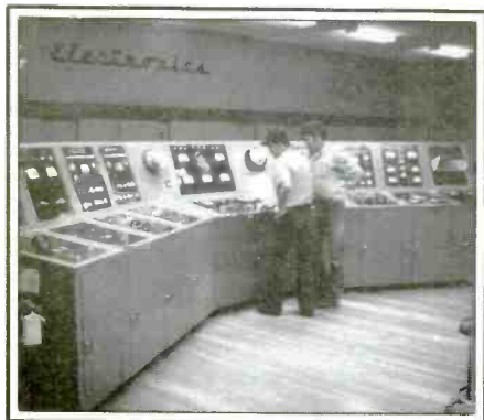
The only station in the world using an AN/FRT-31 transmitter is NAVCOMMU Cutler. Here's how the massive control panel looks.
