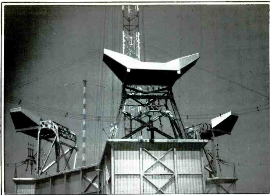
Ice guards are required throughout the system. These protect the helix houses from being damaged by icing.
