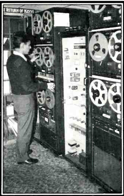
Pfc. Paul Ramirez prepares WFG's automation system.
