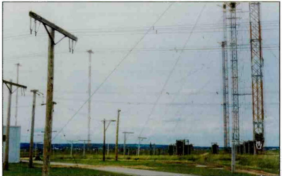
Some of the antennas that radiate from Radio Canada International's Sackville site.
