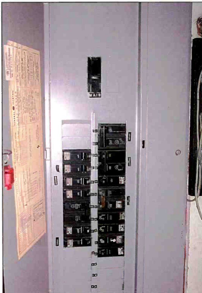
The main circuit breaker panel or fuse box for your home is the first place to start when you're searching out RFI. Switch off one circuit at a time until the interference stops—whatever is causing the problem will be on that circuit.
