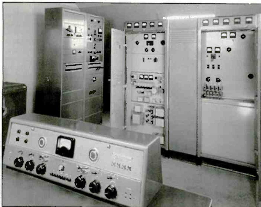
General Electric had broadcast equipment factories (and stations) in several upstate New York cities, including Syracuse. Consequently, the region was particularly flush with GE professional broadcast goods. Shown here is a late 1940s GE FM transmitter installation at one of GE's Syracuse competitor facilities. Key to our story is the 250-watt transmitter at left (with door ajar). The cabinet to its right is an RF amplifier capable of jumping its companion's output to 3 kW. GE FM transmitters in the 250-watt denomination helped start WPTL(FM) and WEAW(FM).
