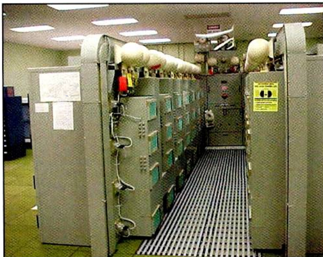
Photo A. LORAN transmitter at the Malone, Florida, station, silent as of February 8, 2010. (USCG photo)
