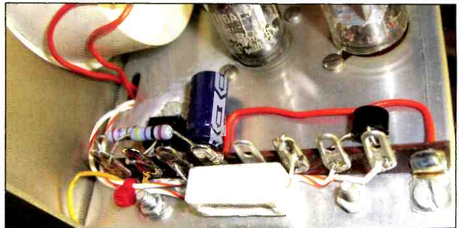
Photo F. The new battery eliminator circuit is mounted on the existing IM-13 sub-chassis. Note that the LM317T is heat sunk to the aluminum chassis to reduce its body temperature; this is optional.
