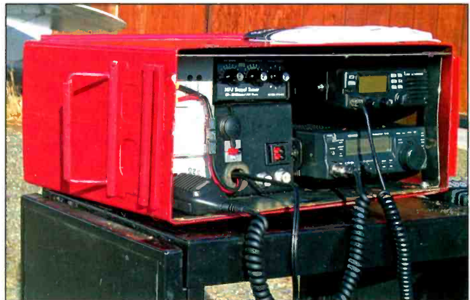
These are "before" and "after" shots of Frank, KLØSW's Bug-Out-Box (BOB). Frank's BOB features a large rechargeable (sealed lead-acid) gelled-electrolyte 20 A/hr battery which is recharged by the A&A Electronics "smart charger." The VHF unit sits above the HF transceiver in the BOB. Deployment is pretty straightforward and Frank can be on the air quickly once he arrives on station.
