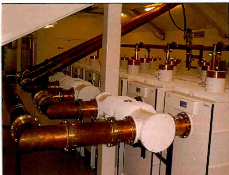
Photo B. Combining network for three analog and three digital FM transmitters.
