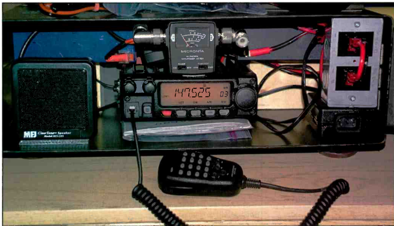
The final fit of the radio, speaker, power/radio patch panel, and dual SLA batteries. The only hardware left to add is the SWR/PWR meter. The power/radio patchpanel on the extreme right allows the operator to charge one battery while using the other one. A second radio (scanner?) can also be added.
