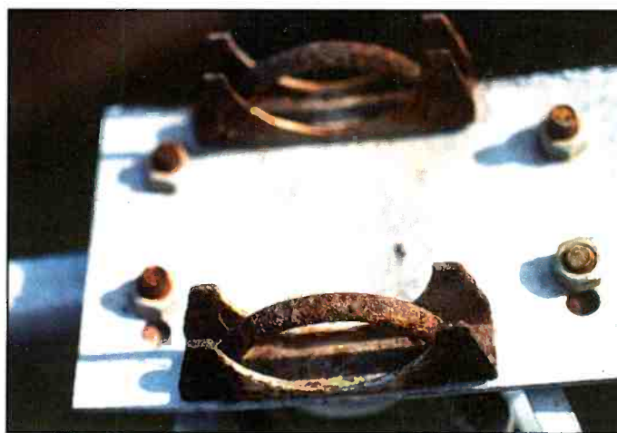
An imported beam didn't use stainless steel hardware.
