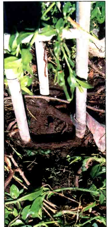
If your tower is in the ground, check for rust! This base fell apart in the storm.
