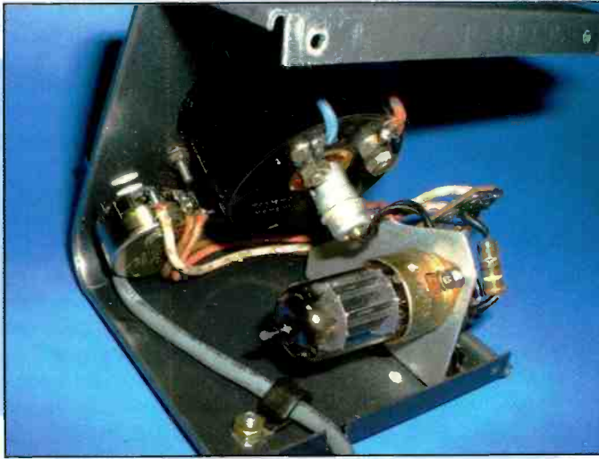
Photo C. Here's a peek on how things were put together. The 12AU7 is mounted on a small-aluminum bracket, along with a terminal strip for mounting most of the components. Photo D better illustrates this area.
