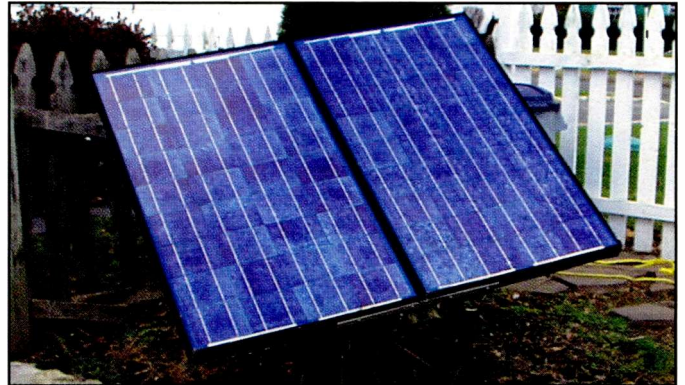
One radio enthusiast put two large solar panels together for his emergency power needs using wood blocks and a post-type mailbox mount.
