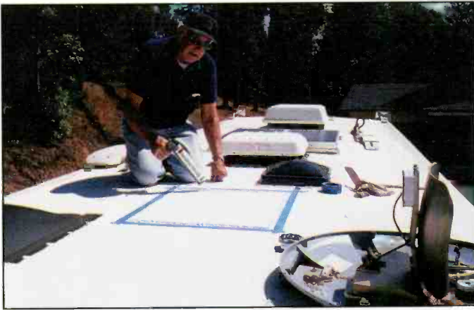
Put down a thick layer of white silicone all the way around the inside of the masking tape, where the antenna will rest.
