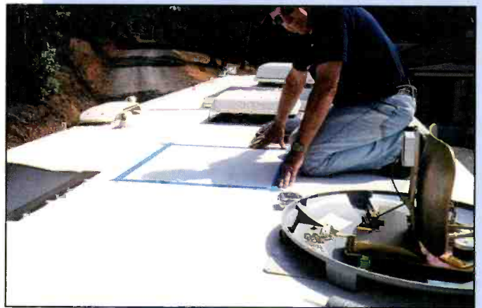
Mask off the exact location and dimensions of the antenna unit. The antenna cover gets removed at this stage.
