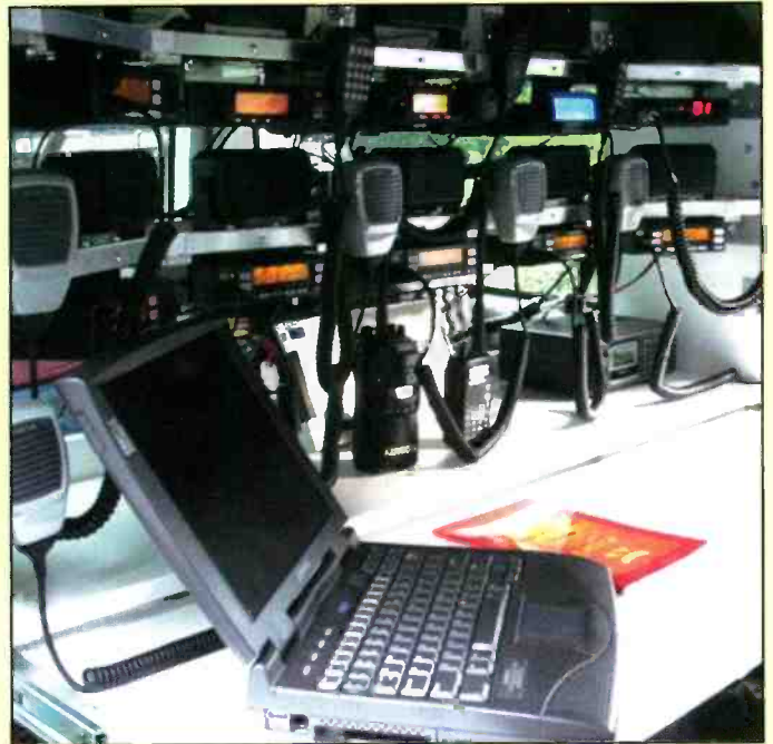
This is an interior shot from the passenger's side of the main operating position. Although crowded, the radio operator can access all bands from 160 meters through 800 MHz from this single location.
