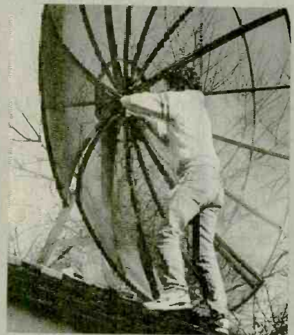
The fourth section is mounted in place. We found it easier to hang it in place before fastening it to its neighboring petals.
