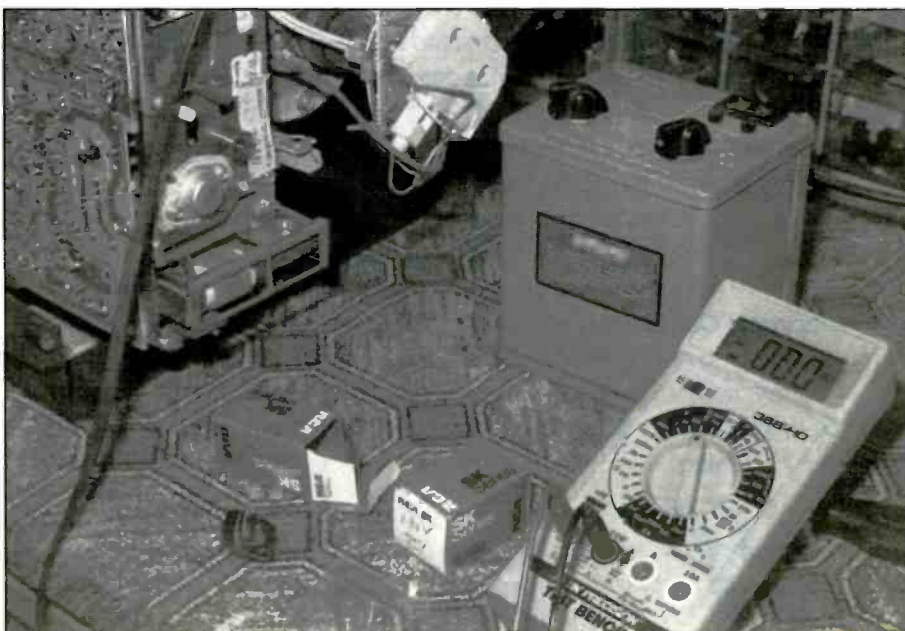
Figure 5. Try to replace the low-voltage regulators with the exact replacement if possible.
