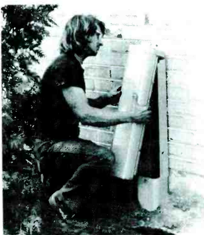
Fig. 14 Metal, weatherproof pedestals outside each building house and protect splitters and amplifiers.
