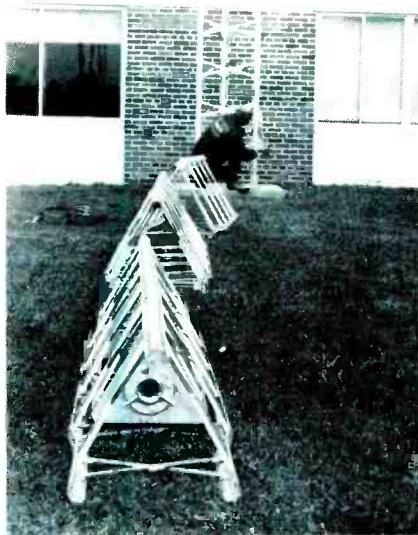
Step 6 After the concrete has cured, and before swinging down the base section for assembly of the tower, recheck the levelness. Use the upper and lower adjustment nuts, if necessary, to make it perfectly level.
