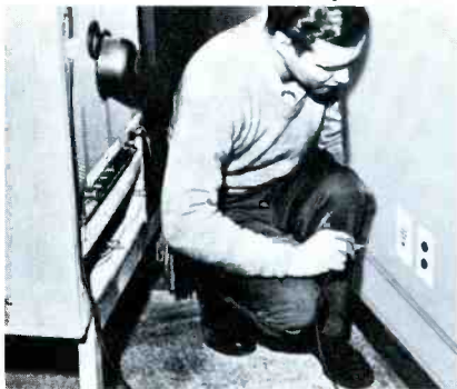
Fig. 5. Individual sets are most easily connected to system via wall plug.
