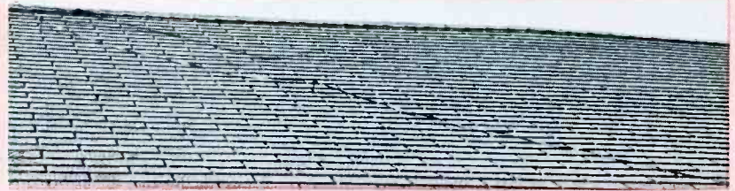
Draping the lead-in across the roof can cause high losses in the line. Proper cabling techniques, using stand-off insulators, remedies this problem.
