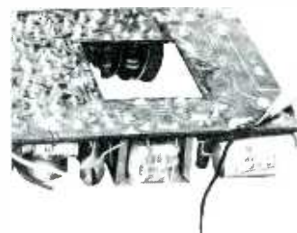
Fig. 3. Blown Conductor and Unbonded Terminal.
