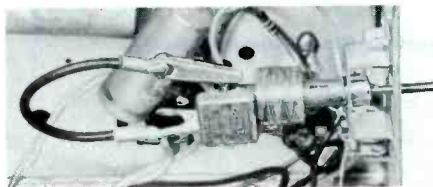
Fig. 3. Ringing Coil Shorted With a Test Lead.
