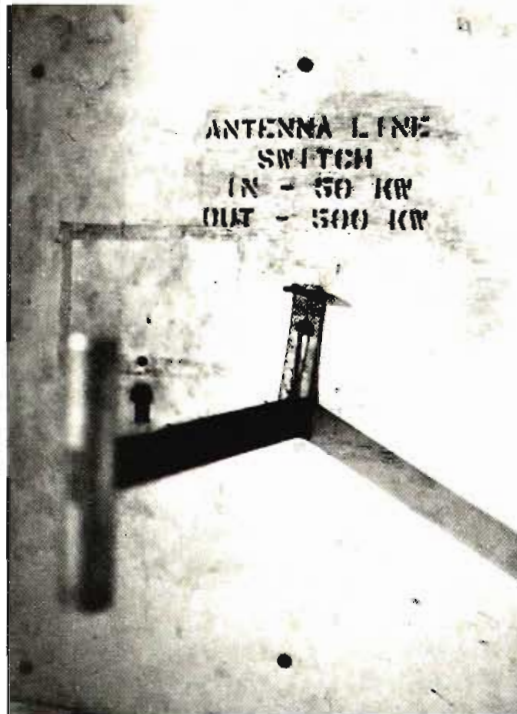
Antenna Line Switch — Transferred tower antenna line from 50 kw Western Electric to 500 kw RCA.
