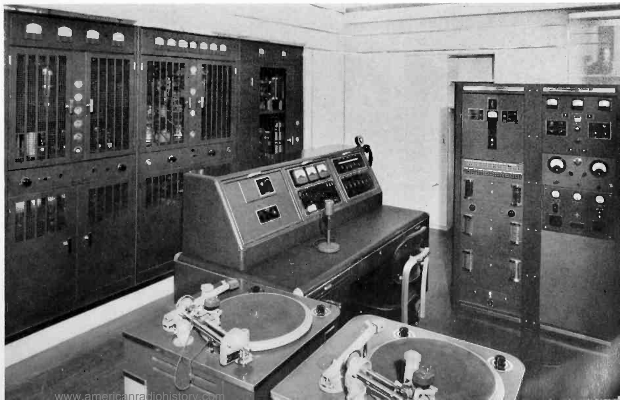
The 5KW transmitter and associate equipment including turntables are Western Electric
