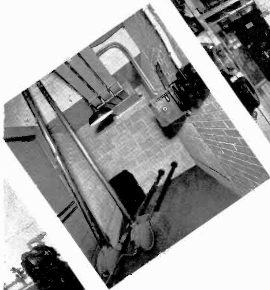
Above panel shows associated equipment for 5,000 watt transmitter. Left to right: Duplicate motor generators used as prime power for transmitting equipment—Concentric transmission lines, coupling unit, tower lighting generator—Entrance room for transmission lines and conduits—Automatic sub-station—Duplicate power control panel and voltage regulators—12,000 volt plate supply for 5 KW amplifier.
