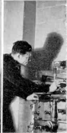
Water pressure controls for the water
