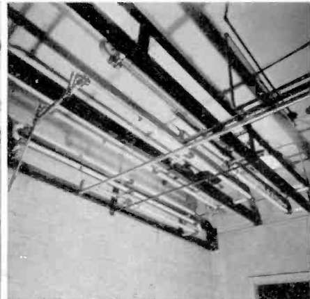
Porcelain tubes mounted on basement ceiling in which cooling water flows.
