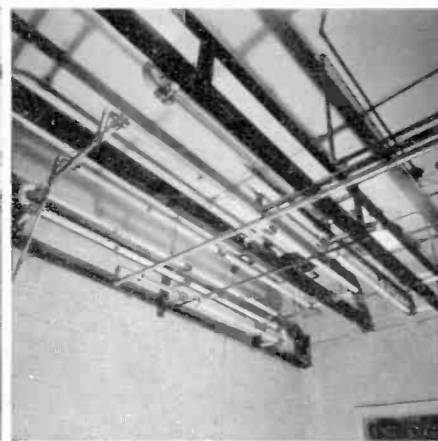
Porcelain tubes mounted on basement ceiling in which cooling water flows.
