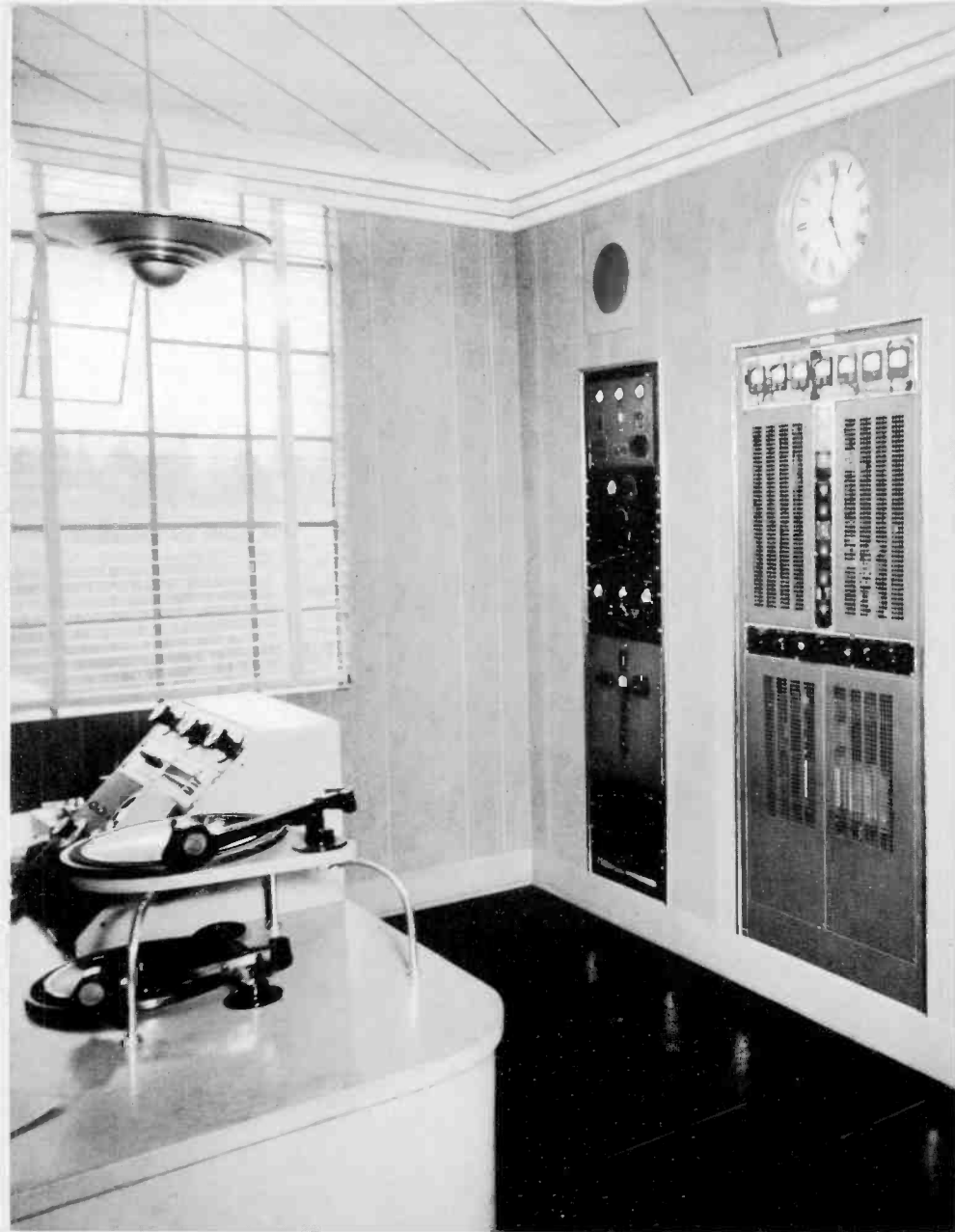
The new Western Electric 310 type transmitter (left) which boosts the station's power from 100 to 250 watts. Dedication programs were heard by New Zealand listeners. The 110A program amplifier is shown at left of transmitter.
