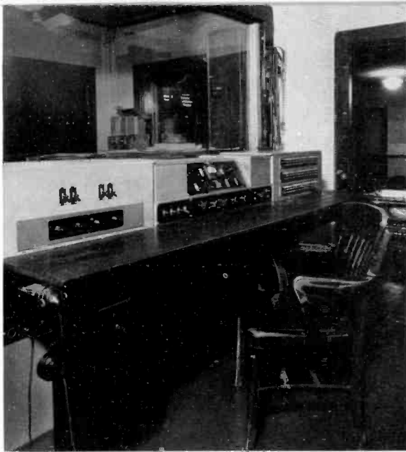
Portion of transmitter room showing studio speech input equipment.
