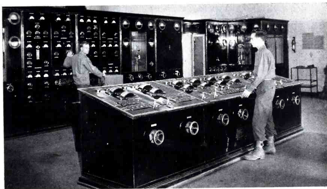
Tuning transmitter at Radio Luxembourg for "Operation Annie", the OSS propaganda program to the Germans. Left, Don V. R. Drenner, chief engineer, and right, Lt. E. A. Rotterman, technical representative.
