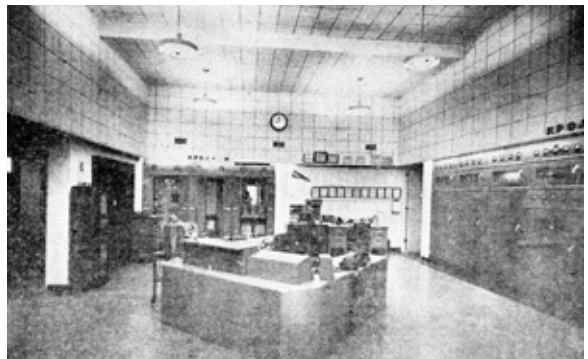
The latest in radio equipment is housed inside transmitter building on Mt. Scott. Seldom seen by outsiders is this view of KPOJ’s 5000-watt transmitter, located several miles from downtown studios.
