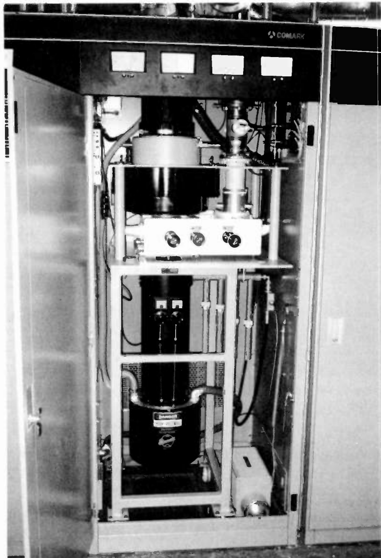
Figure 6 - 30kW Air-Cooled Klystron Tube and Hardware installed in one of WSNS-TV 44 Amplifier Cabinets
