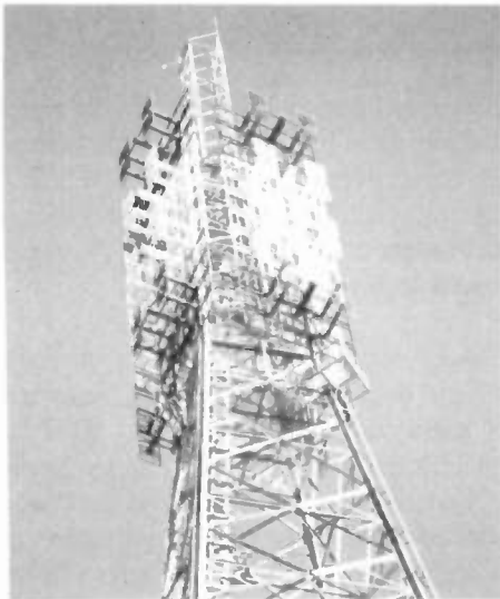
FIG. 8 - VHF NEW ZEALAND TV ANTENNA UHF TV OMNI ANTENNA ON ROTATING TOWER
