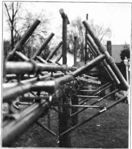
Figure 7 - FM directional antenna system in final testing.
