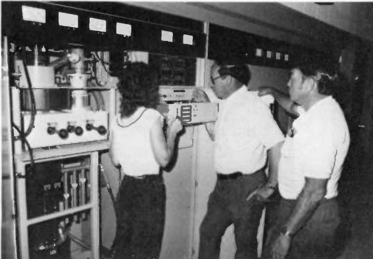
Figure 12 - WABW Staff Members Examining Comark 120kW Klystrode Equipped Transmitter - Pelham, Georgia
