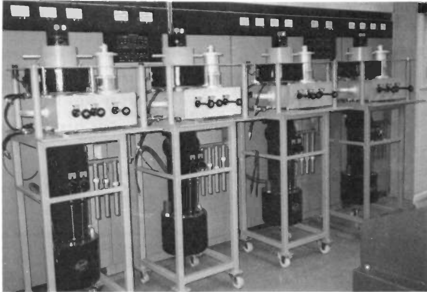
Figure 3 - Three Klystrode Tubes plus Spare ready for installation at Wrens, Georgia
