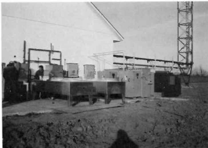
Figure 20 - Dual Heat Exchangers and Dual Power Supplies which add redundancy to the transmitter system at WIIB-TV
