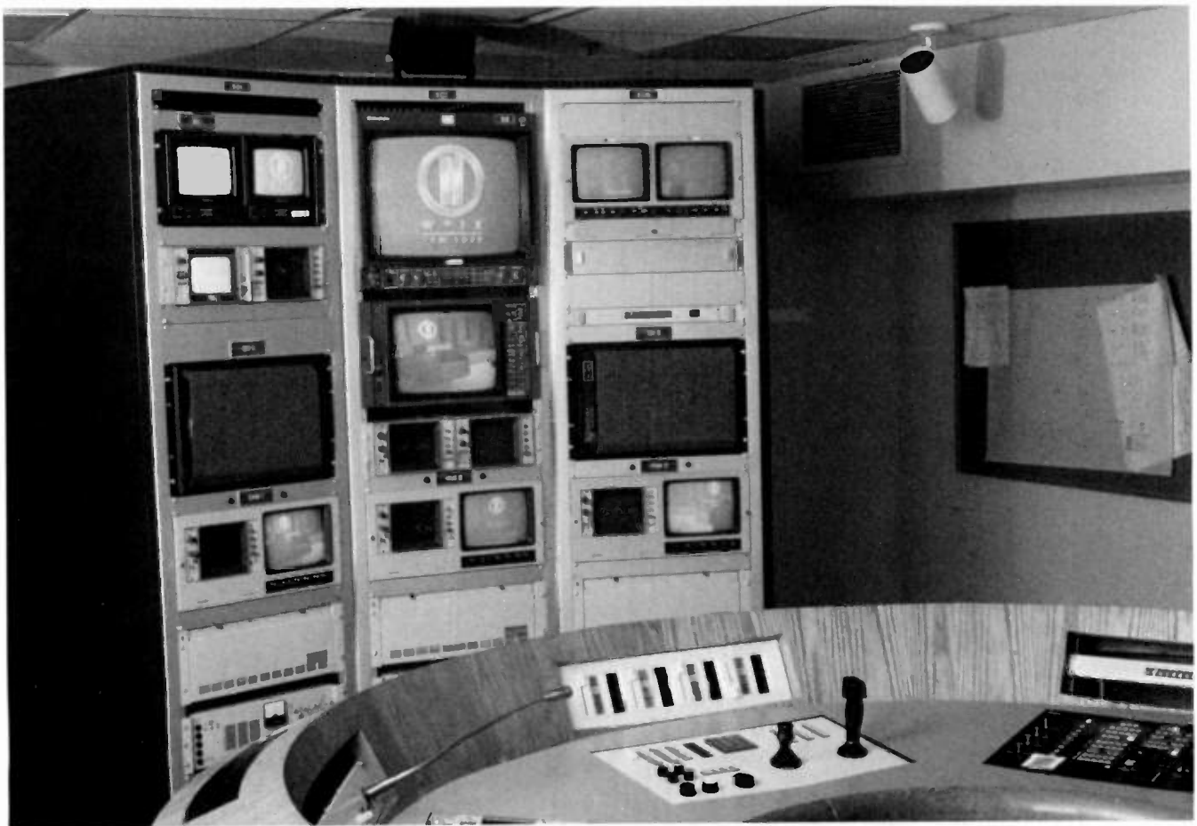
WPIX VIDEO CONTROL ROOM
