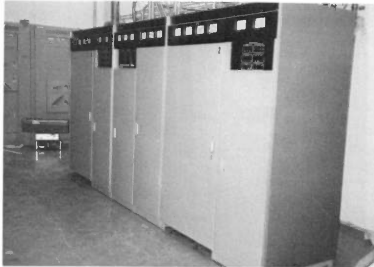
Figure 17 - 80kW Transmitter installed at WIIB-TV - Bloomington/Indianapolis
