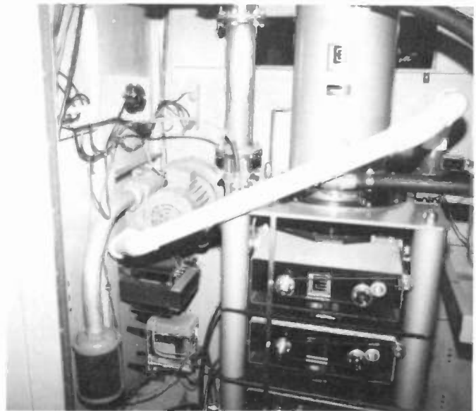
View shows high velocity blower used to cool klystron and circuit assembly. PVC pipe is used as an air duct.
