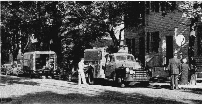
FIG. 5-31. Person-to-Person television remotes usually require more electric power than is available in the homes visited. Consequently, a special temporary electric service is needed. A power-company crew is providing this service at a Georgetown, Washington, D.C., residence.
