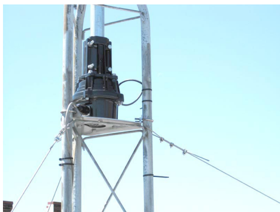
Expertly installed at W7MRE (The American Museum of Radio and Electricity in Bellingham, WA), this Yaesu G800-SA rotator (a best buy in this year's MT Buyer's Guide), rated for a beefy 17 square feet of wind load) loafs along while aiming the club station's Traffie Technology Hex-Beam antenna, which has a wind-load rating of less than 5 square feet. Note the rotator shelf (see text). (Photo by, and courtesy of, Phil Terzian, AE6K.)
