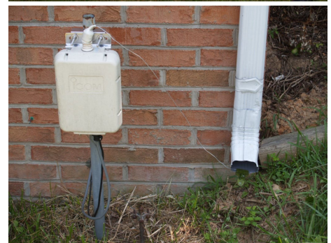
In 2010, during a year of casual operating and rather poor overall propagation, Bill Mabry N4QA, of Radford, Virginia, made 560 contacts on 160 through 6 meters, 558 of which were at 5 W or less, using this downspout as his antenna! Fed with an ICOM AH-4 auto-coupler for lightning-fast band changes, Bill calls the antenna GADS, short for Gutter and Down Spout. In addition to working QRPDX on four continents, Bill worked all states except Hawaii and most Canadian provinces. If Cycle 24 perks up in 2011, look for Bill to be busting pileups in every direction! (Photos courtesy: N4QA)
