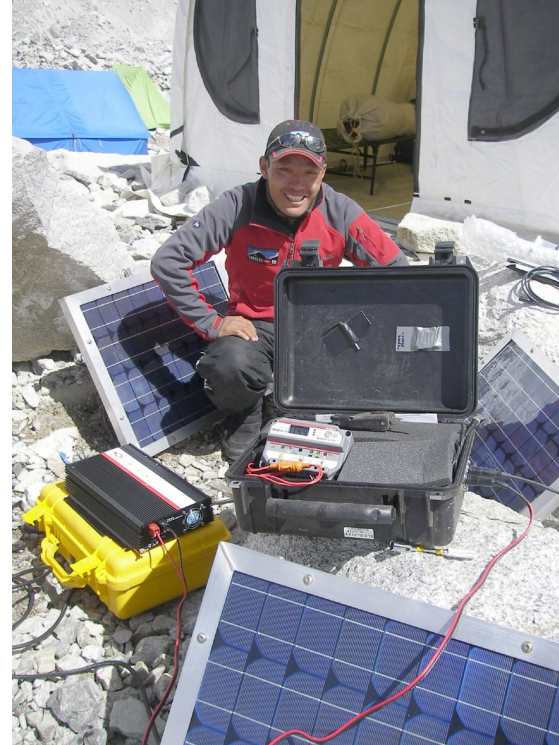
Solar panels and charge controller at base camp on 2008 Everest expedition.
