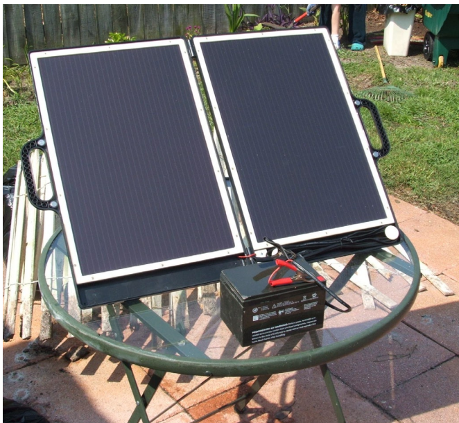
Solar panels connected to charge a 12 volt battery can be used to provide power to radios in an emergency
