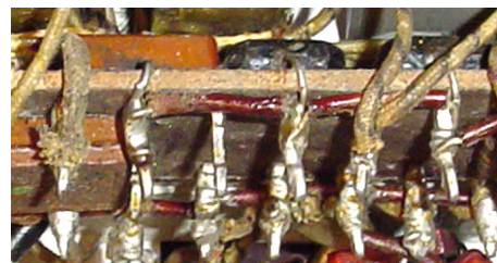
Inaccessible capacitors (top part of picture) were removed from the circuit by cutting their leads where they wrapped around the top of the resistor board. This made it possible to install new caps on the other side of the board (see text).
