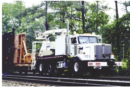
A Norfolk Southern Brandt unit maneuvering railcars with track components into place for unloading by crane. Note that the unit is equipped with a hydraulic arm that can be used either as a lightweight crane or as a cherry-picker to lift personnel to work on lineside equipment.
