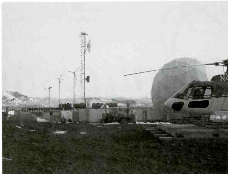
View of the Black Island Telecommunications Facility. The dome houses the 11-meter dish for the satellite to the U.S. Three of the four wind generators are visible, the roof of the buildings are covered with solar panels. The fuel tanks in the background are used for the backup generators. The microwave dishes connect the communications equipment here to McMurdo (about 20 miles away).
