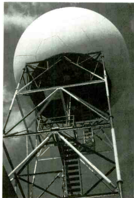
The NEXRAD radome. Inside is a 28 foot parabolic dish with a 360 degree vision out to 250 miles.
