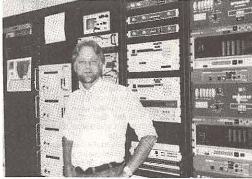
Jerry Lopez, a WSHB engineer, in front of the control room rack.
