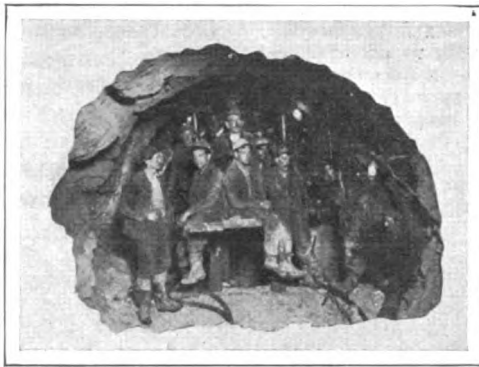
A VIEW IN THE TWELVE-FOOT TUNNEL, SHOWING THE LABORERS OR "TUNNEL STIFFES" AS THEY ARE KNOWN
