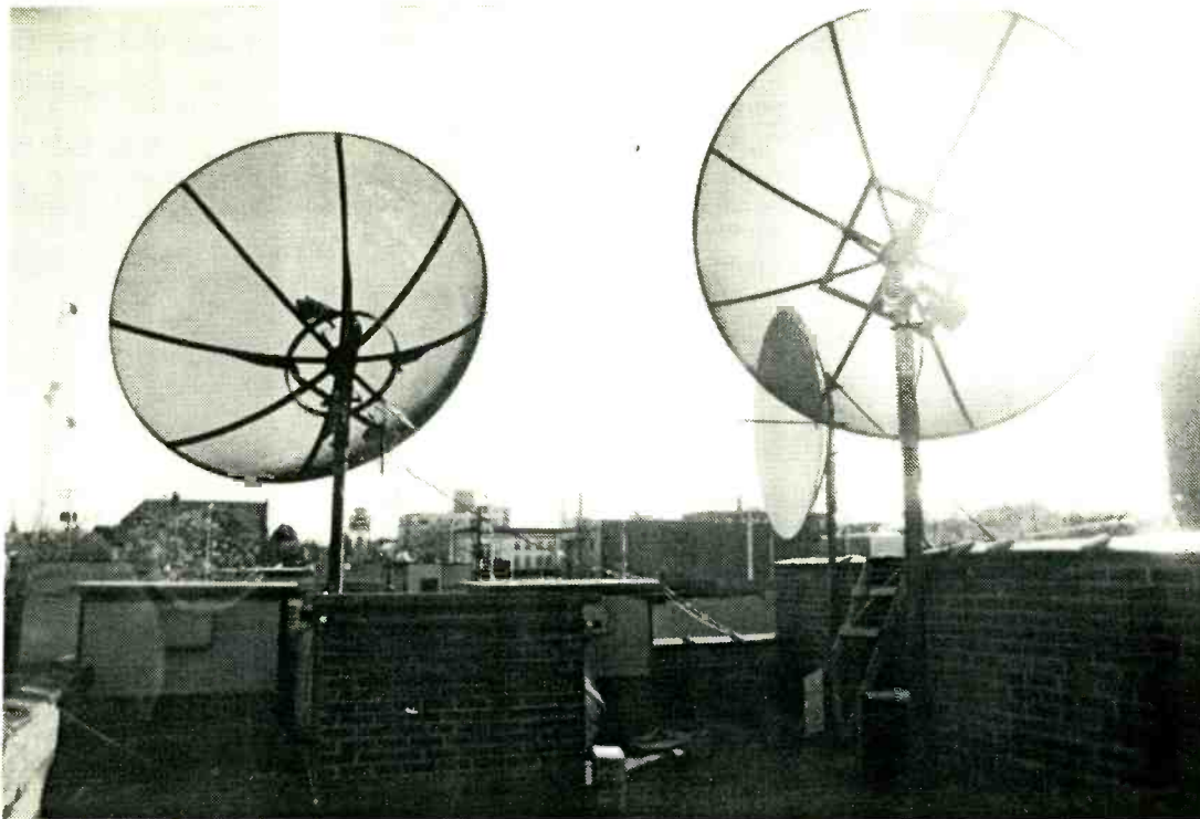
Two ten-foot Winegard mesh satellite dishes with power operator moving systems on the Sioux Falls roof. Old, beat up, eight-foot Andrew dish, white one on right, is used to carry STL signal two miles to transmitter on channel 23.
