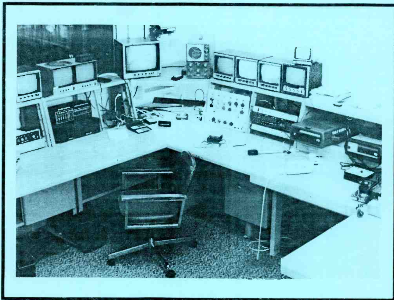
Start of the Sioux Falls Studio Control Room
