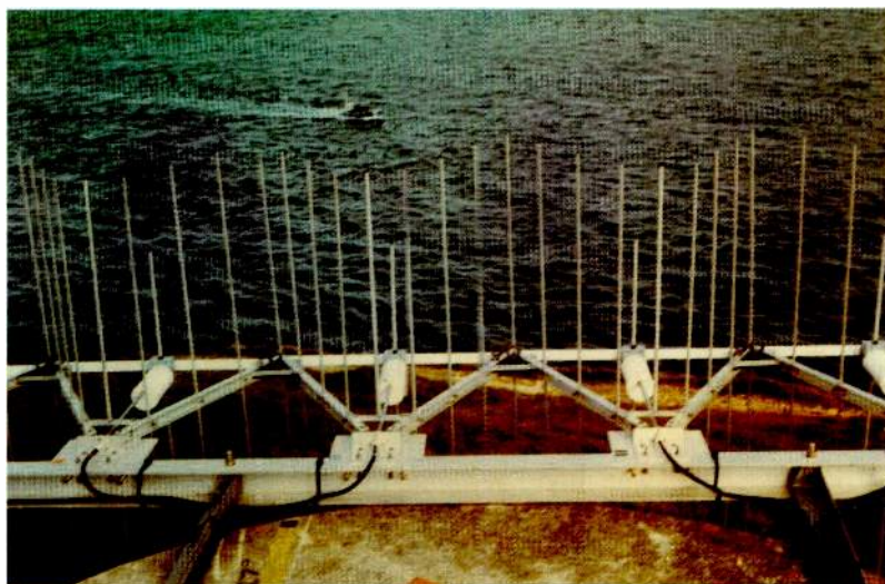
Radio lighthouse antenna mounted on the fog signal housing at Anvil Point, England.
