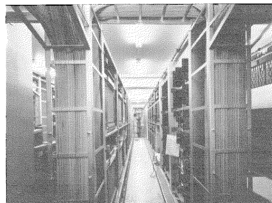
Figure 10—View of 2 of the 21 rows of equipment in the Oslo automatic toll exchange.
